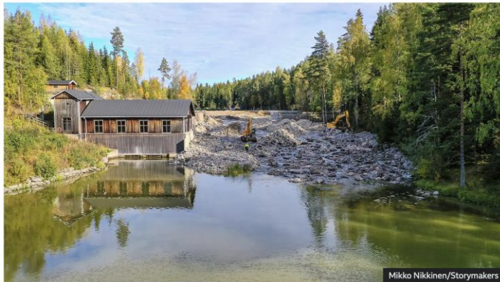
Dam removal is a meticulously planned and lengthy engineering work (Credit Mikko Nikkinen/Storymakers)
